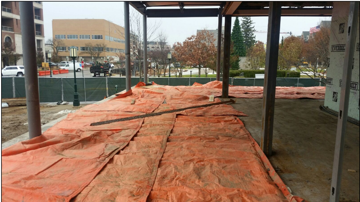
The elements that make up concrete form a chemical reaction that creates heat. Once the concrete is poured and cures for a few hours, concrete blankets are placed on the concrete. These blankets help to trap in the heat and assists the concrete in fully curing over the course of a week or so.
