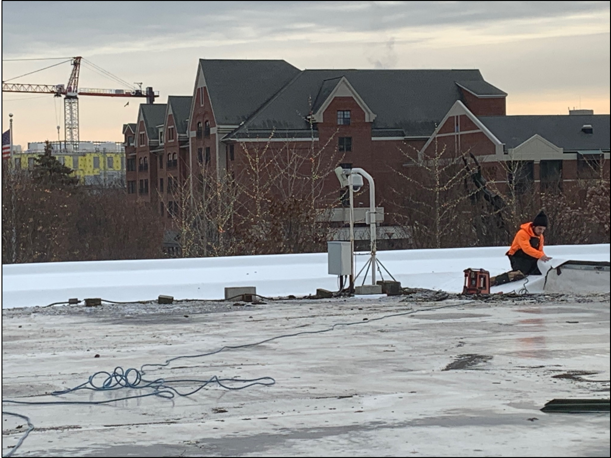
The roof over the Youth Room addition was installed on December 12 (in 18 degree weather).
