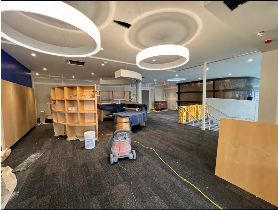
View of new information desk and entry staircase from book sorter room
